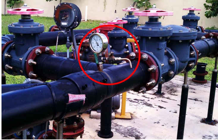
Figure 4: S.E. Step-up Station Sampling Port
